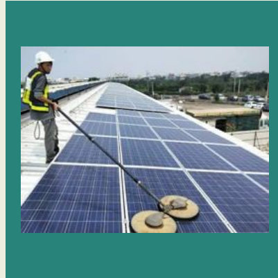
Solar Panel Cleaning System
